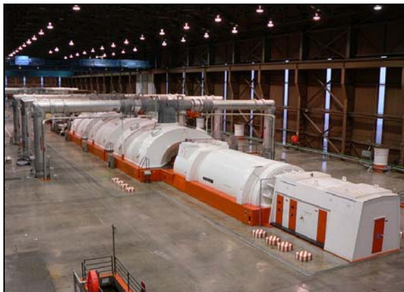
Fig. 7: Steam Turbine at a Nuclear Facility
